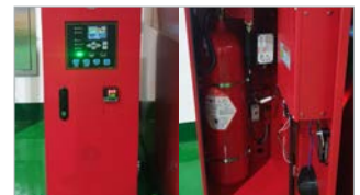
④ CO 2 Fire Extinguisher System
